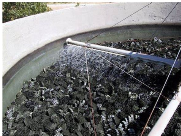
Figure 12. Discs in bacterial bed [online]. Source: https://th.bing.com/th/id/R.55c3fe2266a8fcab38b9534ad9dda10e?rik=fiC9BsLfFk2NfQ&riu=http%3a%2f%2fwww.aguasresiduales.info%2fmedia%2fimages%2fckfinder%2fuserfiles%2fimages%2f1012.JPG&ehk=SLHn0C5XQgHwJRSEdYShXyAHzVZVdrNznvN8bavNUiw%3d&risl=&pid=ImgRaw&r=0 [Accessed on: 2026]
