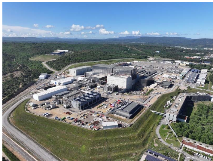
Figure 3. Image: Drone view of the ITER tokamak and construction site. 14-05-2025 - Photo: ITER Organization/EJF Riche.
